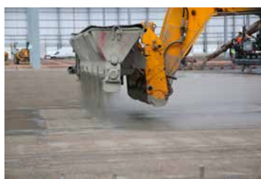
Top: Close-up of SFRC. Middle: Steel fibres are added to the concrete. Above: Dry shake topping is applied.
